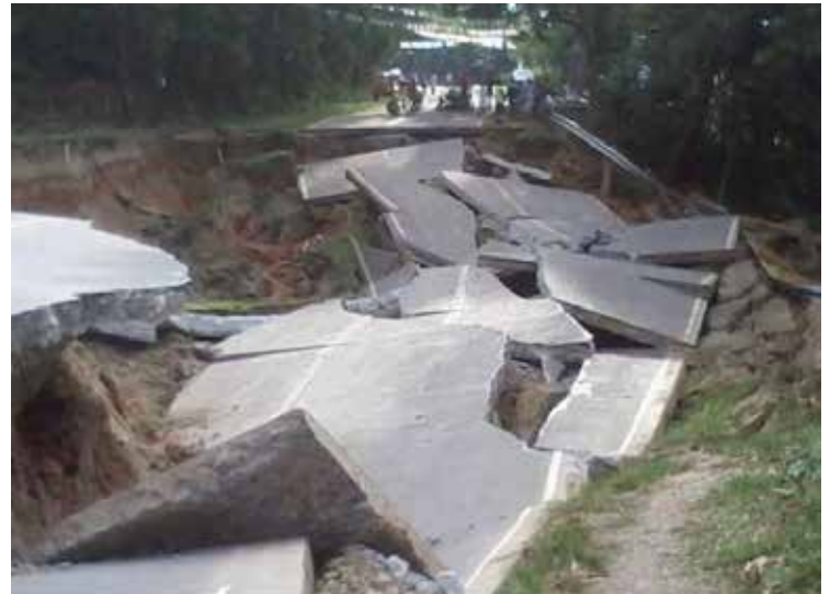
The Bohol earthquake destroyed many roads, bridges and hospitals in Bohol.
