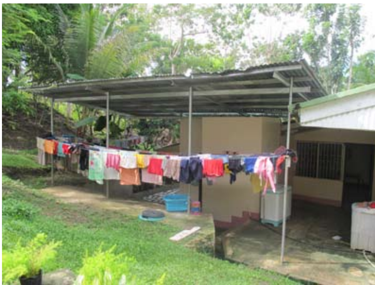
The new overhang at the Sunshine Home allows wet laundry to dry on rainy days.
